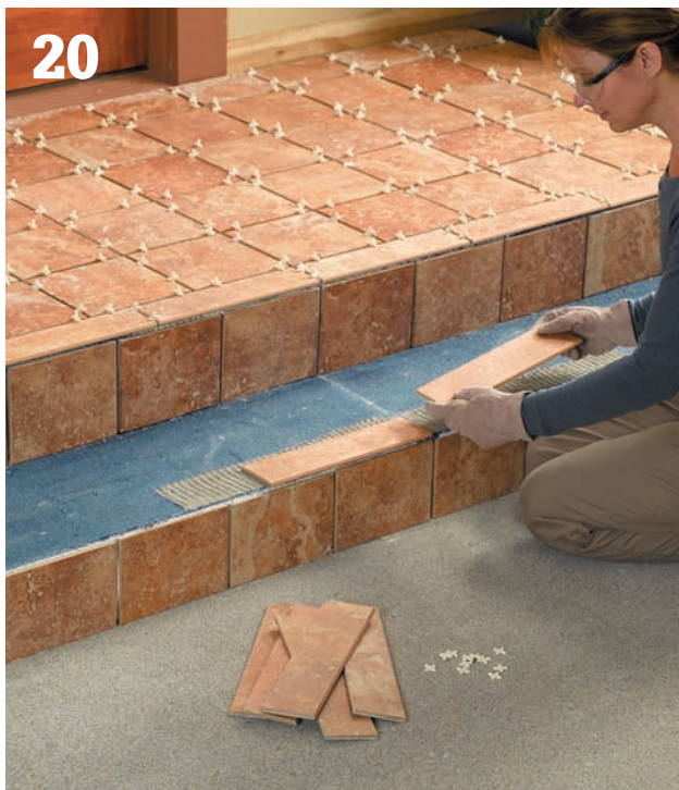
20 Install tiles on the stair treads, starting at the top tread and working your way downward. Set a bullnose tile on each side of the centerline and work your way toward the sides, making sure to conceal the step-side tiles with the tread tiles.
