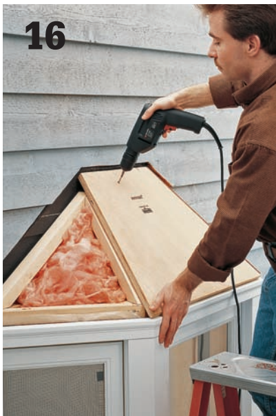
16 Fill the empty space inside the roof frame with loosely packed fiberglass insulation. Screw the sheathing back onto the roof frame using 2" utility screws.
