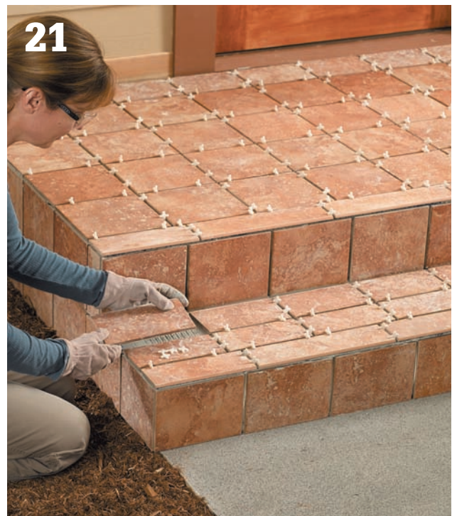
21 Fill in the field tiles on the stair treads, being sure to leave a gap between the back tiles and the riser tiles that's the same thickness as the other tile gaps.
