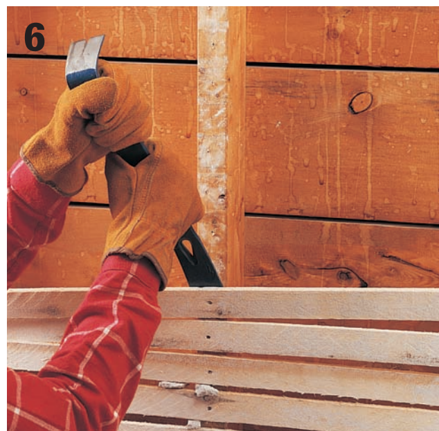
6 Remove the lath from the studs using a pry bar. Pry away any remaining nails, and remove any vapor barrier and insulation.
