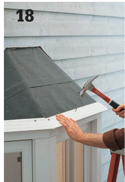
18 Cut drip edges with aviation snips, then attach them around the edge of the roof sheathing using roofing nails.
