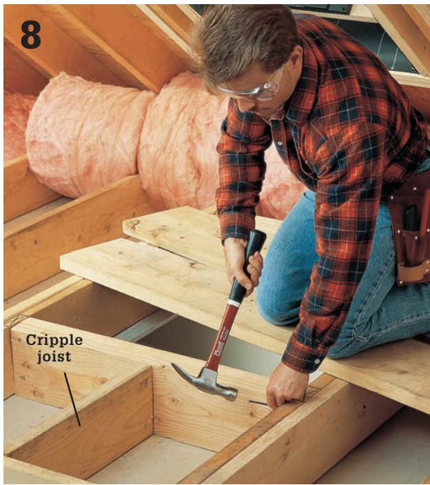
8 Install the double header and double sill, anchoring them to the king joists and cripple joists with 10d nails. The inside edges of the header and sill should be aligned with the edge of the ceiling cutout.
