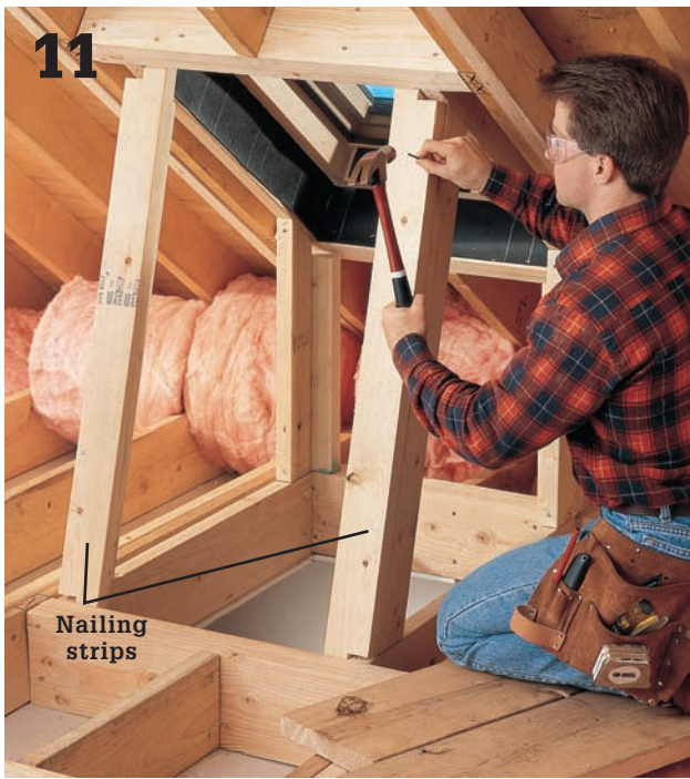
11 Attach a 2 × 4 nailing strip to the outside edge of each corner post to provide a nailing surface for attaching the wallboard. Notch the ends of the nailing strips to fit around the trimmers; a perfect fit is not necessary.
