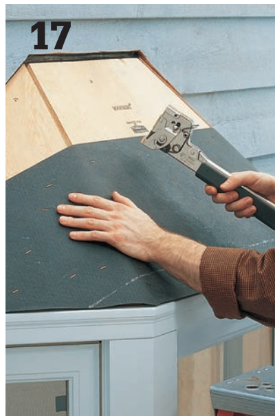
17 Staple asphalt building paper over the roof sheathing. Make sure each piece of building paper overlaps the one below by at least 5".
