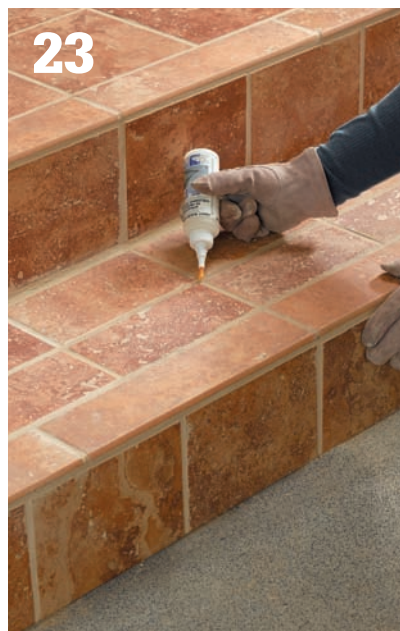
23 After a few weeks, seal the grout lines with an exterior-rated grout sealer.
