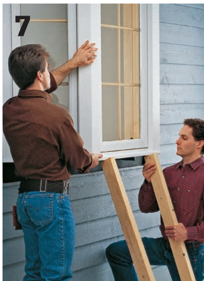
7 Check the window unit to make sure it is level. If necessary, drive shims under the low side to level the window. Temporarily brace the outside bottom edge of the unit with 2 x 4s to keep it from moving on the braces.
