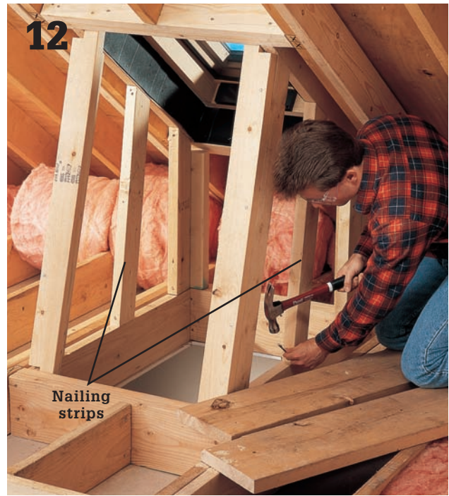
12 Install additional 2 × 4 nailing strips between the corner posts if the distances between posts are more than 24". Miter the top ends of the nailing strips to fit against the rafter trimmers.
