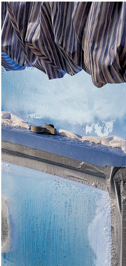
Condensation or frost buildup on windows is a sign of poor weather stripping and an inadequate storm window.
