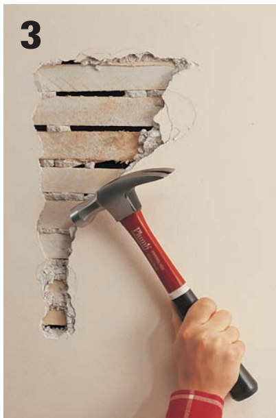
3 Beginning at the top of the wall in the center of the planned opening, break up the plaster by striking the wall lightly with the side of a hammer. Clear away all plaster from floor to ceiling to within 3" of the marked lines.
