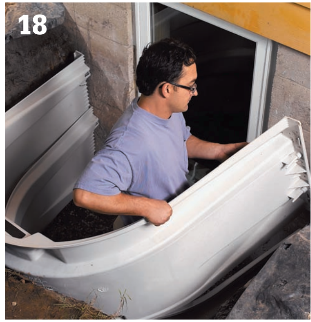
18 Stack the second well section on top of the first, and connect the two with the appropriate fasteners.
