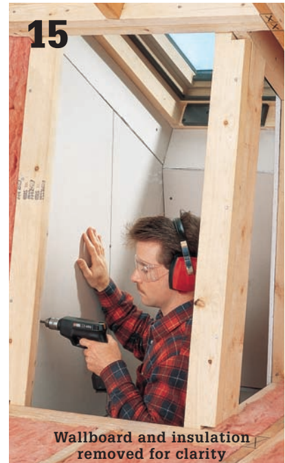
15 Finish the inside of the shaft with wallboard (pages 288 and 289). Tip: To reflect light, paint the shaft interior with a light-colored, semigloss paint.
