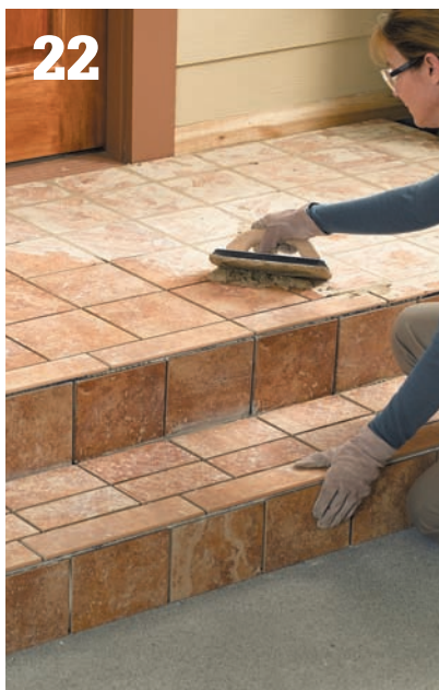
22 Let the thinset mortar cure for a few days, and then apply grout in the gaps between tiles using a grout float. Wipe away the grout after it clouds over. Cover with plastic, in the event of rain.
