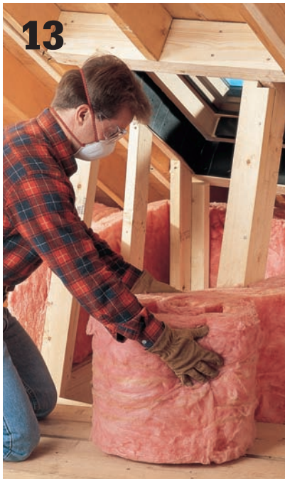
13 Wrap the skylight shaft with fiberglass insulation. Secure the insulation by wrapping twine around the shaft and insulation.
