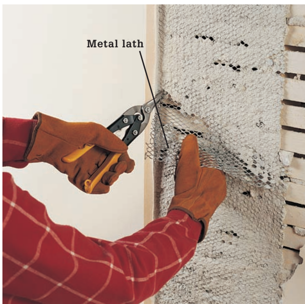
Variation: If the wall has metal lath laid over the wood lath, use aviation snips to clip the edges of the metal lath. Press the jagged edges of the lath flat against the stud. The cut edges of metal lath are very sharp; be sure to wear work gloves.
