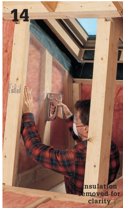
14 From inside the shaft, staple a plastic vapor barrier of 6-mil polyethylene sheeting over the insulation.
