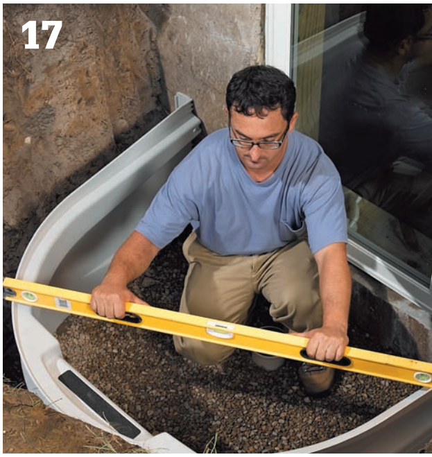
17 Set the bottom section of the well into the hole, and position it evenly from left to right relative to the window. Adjust the gravel surface to level the well section carefully.
